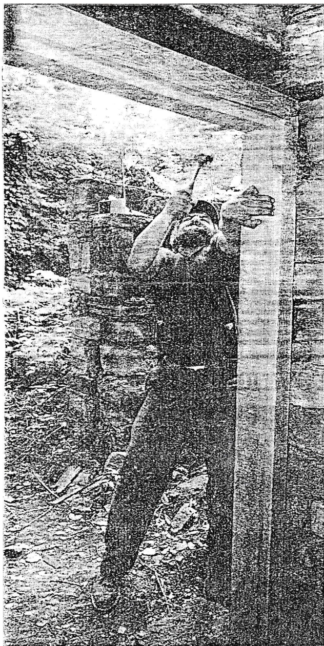
GARRY BROWN Gazette Photographer James D'Agostino drives a pin into a new door frame as part of the restoration of the entryway of the 1750 Nellis Tavern.
